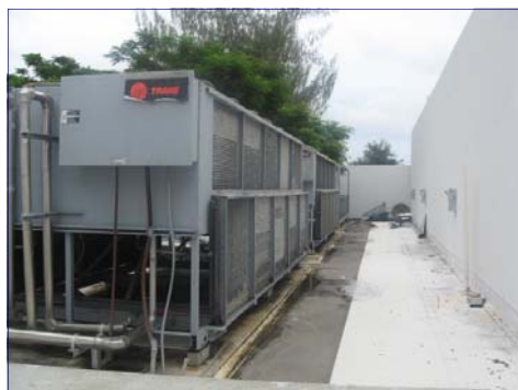
Condensing unit coils soon to be replaced at the Guma Hustisia.
